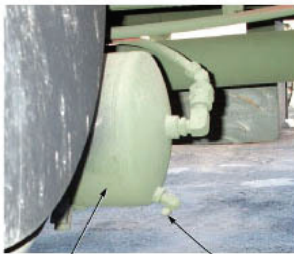
AIR RESERVOIR NO. 2 (OTHERS SIMILAR)
